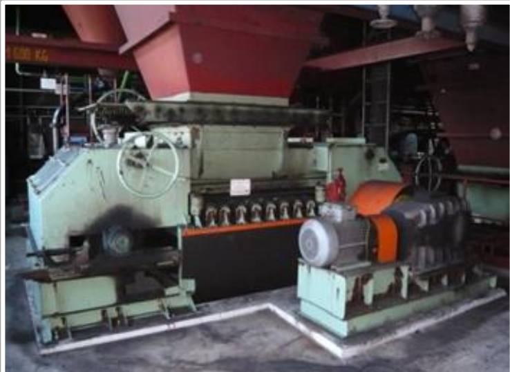
Belt discharge, Paskov Mine, OKD Q = 120 – 150 t/h
