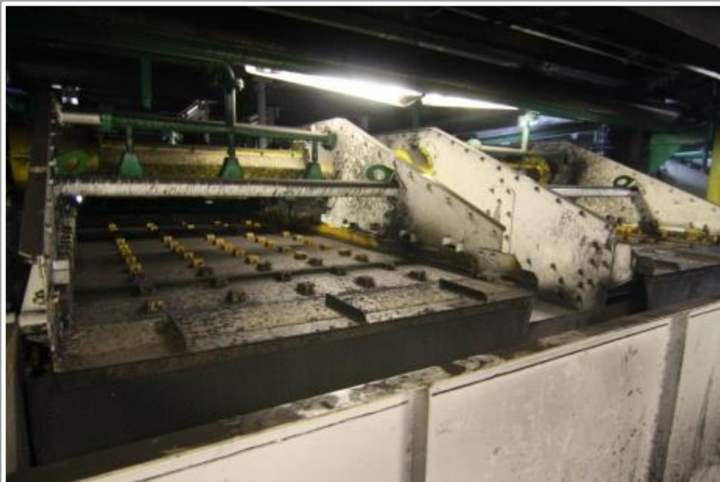
Vibrating screeners, ČSM Mine, OKD Q = 80 t/h
